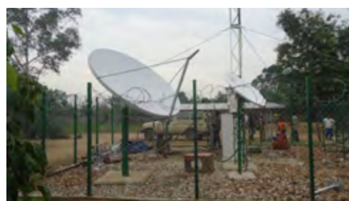
Image: Secure installation of solar-powered, satellite-enabled, mobile base station - Rascomstar
